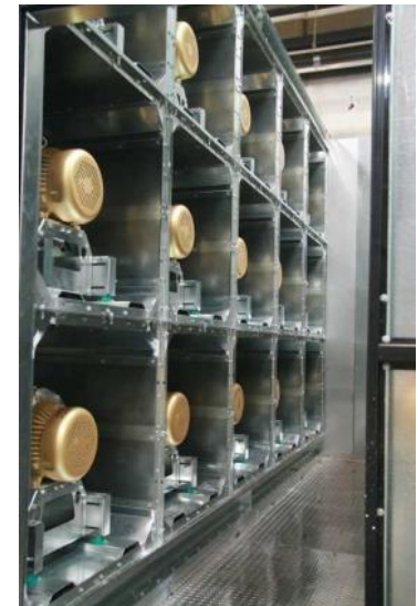
Fanwall AHU (TRIP)
