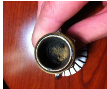
Failed Sprinkler Head (Illinois, 12 year old system)
