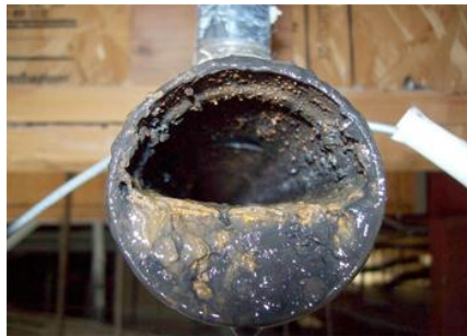
50% Blockage (California, 5 year old system)
